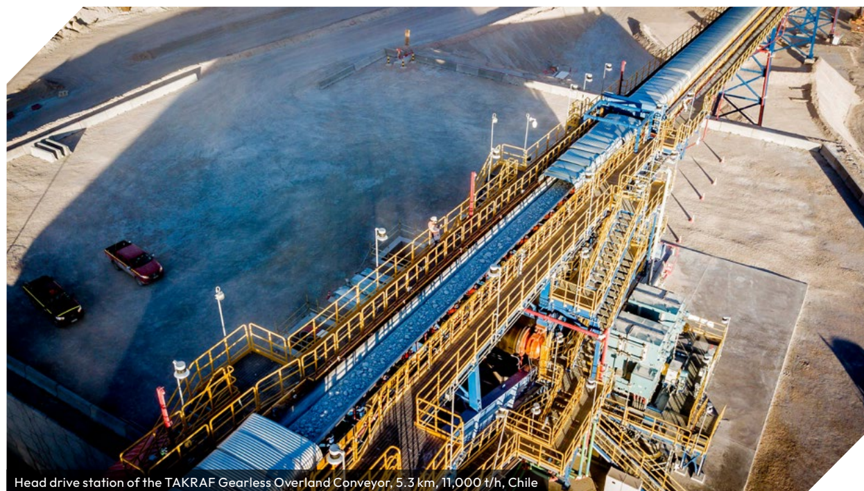
Head drive station of the TAKRAF Gearless Overland Conveyor, 5.3 km, 11,000 t/h, Chile
