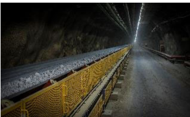
Caption: First ore conveying on the 7 km long TAKRAF gearless underground conveyor system at Chuquicamata in Chile.
