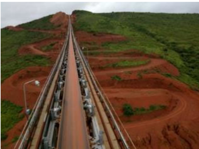
Caption: A very undulating terrain typified the path of the 19 km overland conveyor moving bauxite ore from the mine to the Utkal alumina plant in India
