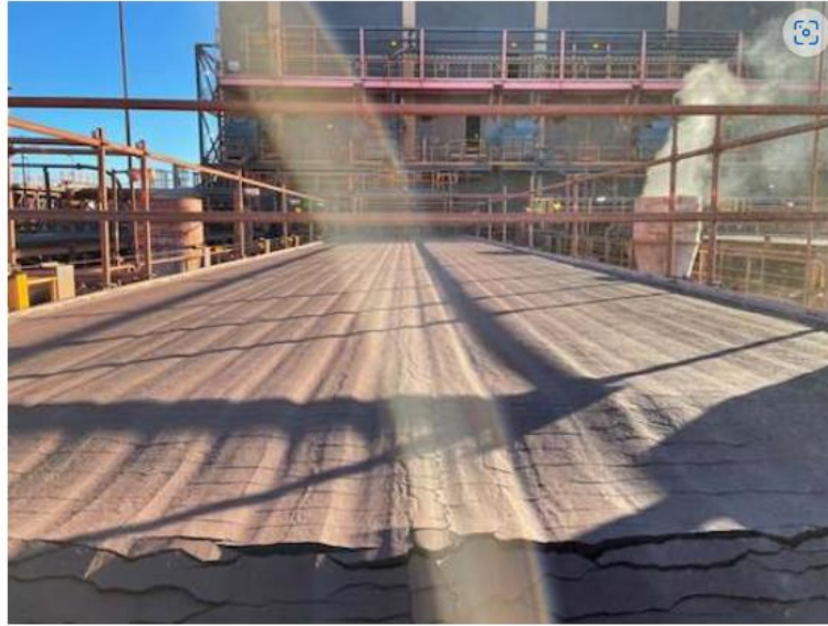
Before the old cake consistency feeder was installed.
