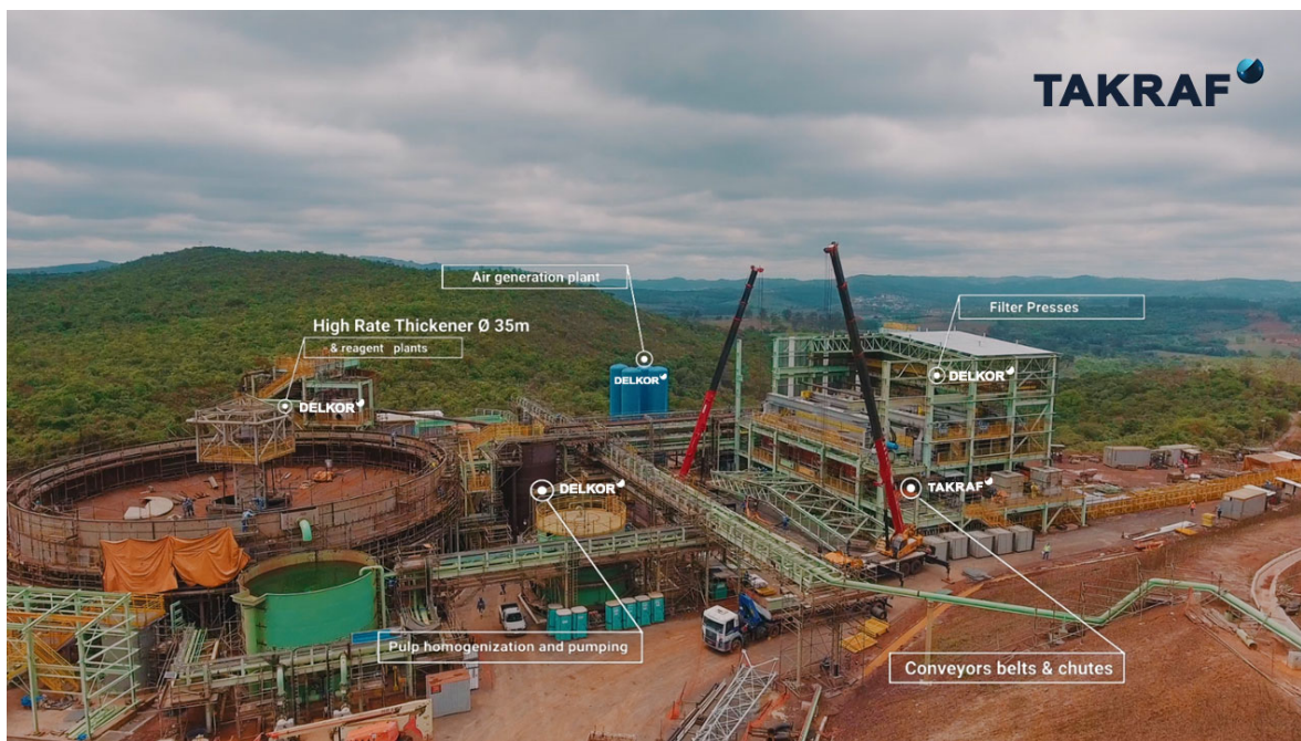
DST system under construction for the safe and effective handling of iron ore process tailings recently supplied by TAKRAF Brazil to Mineração Usiminas.
